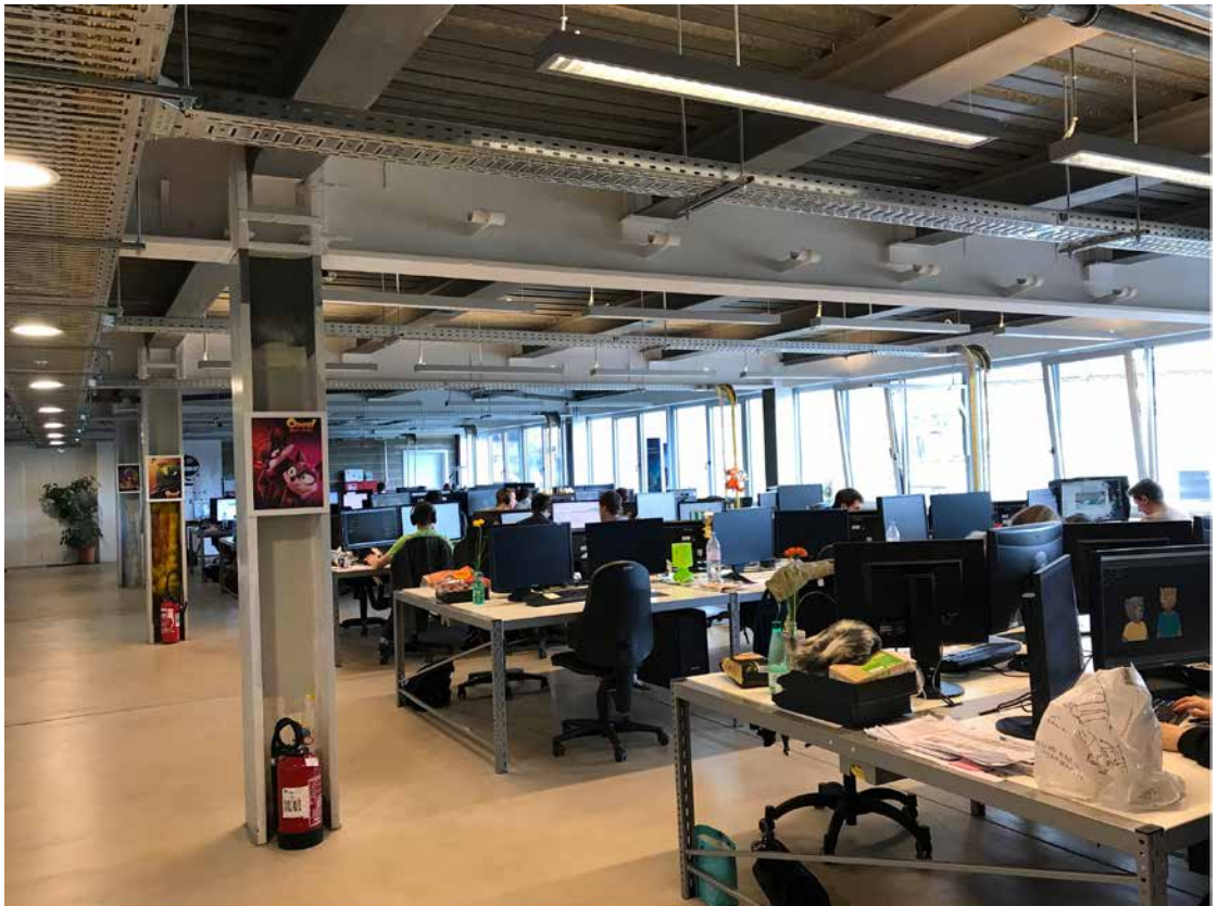
Fig. 22: Open office for 3D software developing company on Level 3, the steel structure with HE300M - columns and HE600B - beams being visible and not protected by any insulation.
