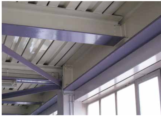
Fig. 4: Beautifully painted steel elements on level 3 existing since 1970 and kept as such unprotected during retrofitting.
